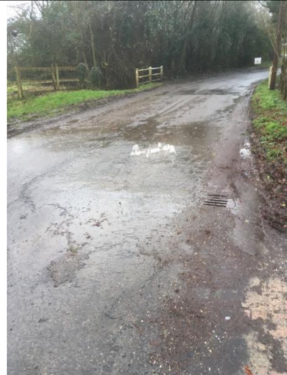
Fernham Road – Jan 21 – note sewer proximity to road drain
